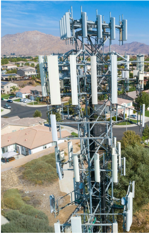
Close-up aerial of a cellular wireless mobile data tower with a neighborhood surrounding.
