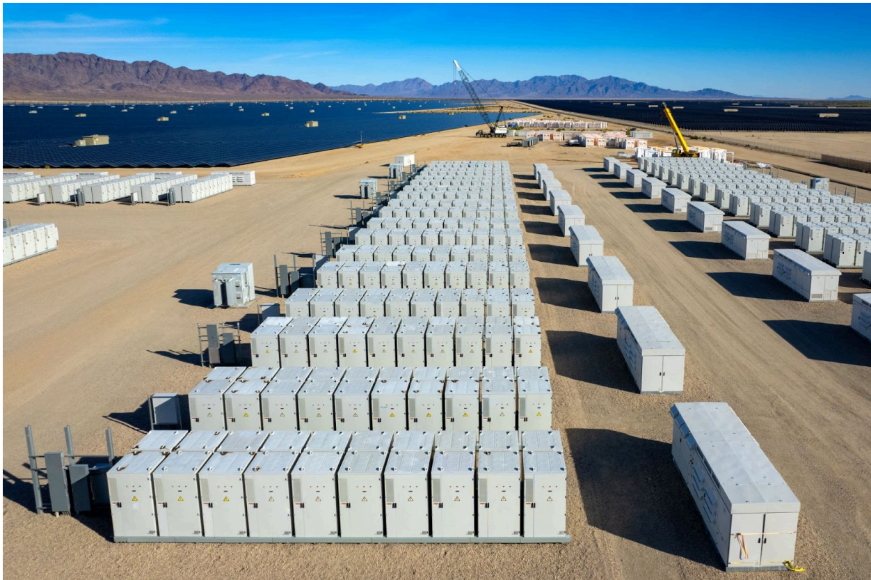
Aerial view of solar farm battery storage units.
